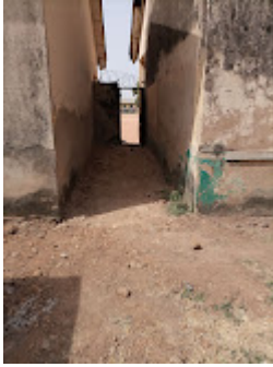
Toilet area before interlocks 1_compress80.jpg 775K
